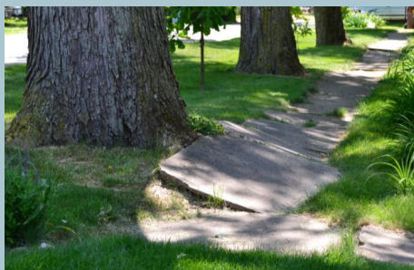
Grade F – Not present, broken, and/or impassable.
