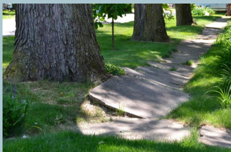
Grade F – Not present, broken, and/or impassable.
