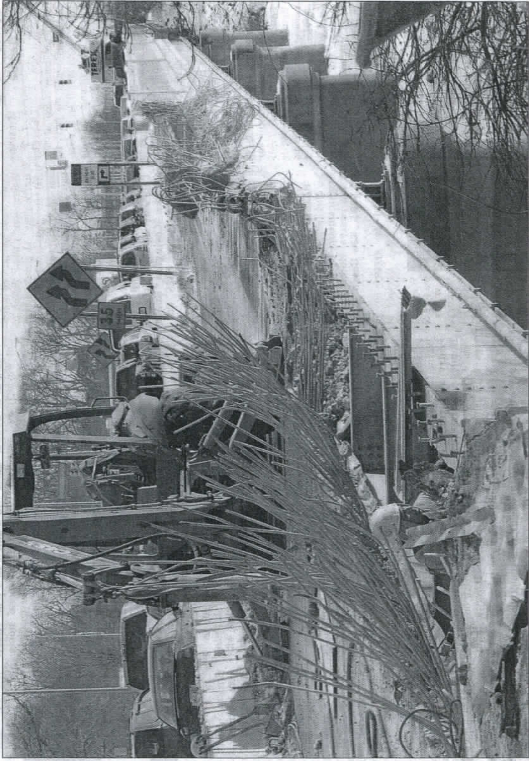
Eastbound traffic is backed up Tuesday as work begins to extend the Rivergreenway across the St. Joseph River via the Coliseum Boulevard bridge near North Anthony Boulevard. The work is expected to be complete in early April.
